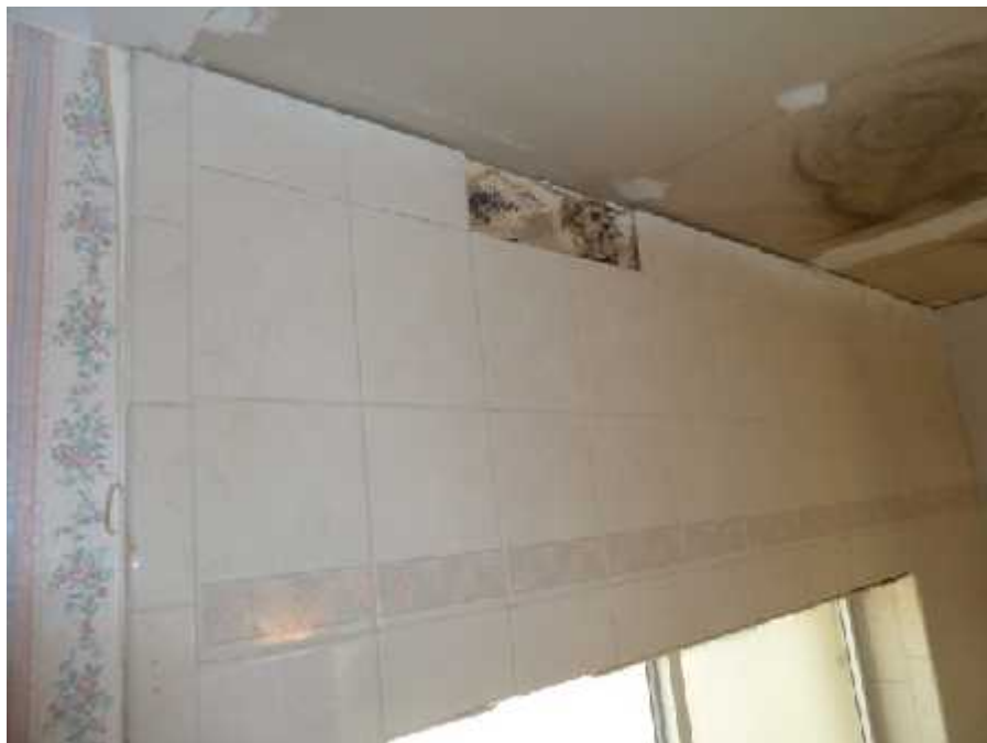
Damage also Behind Shower Tile
