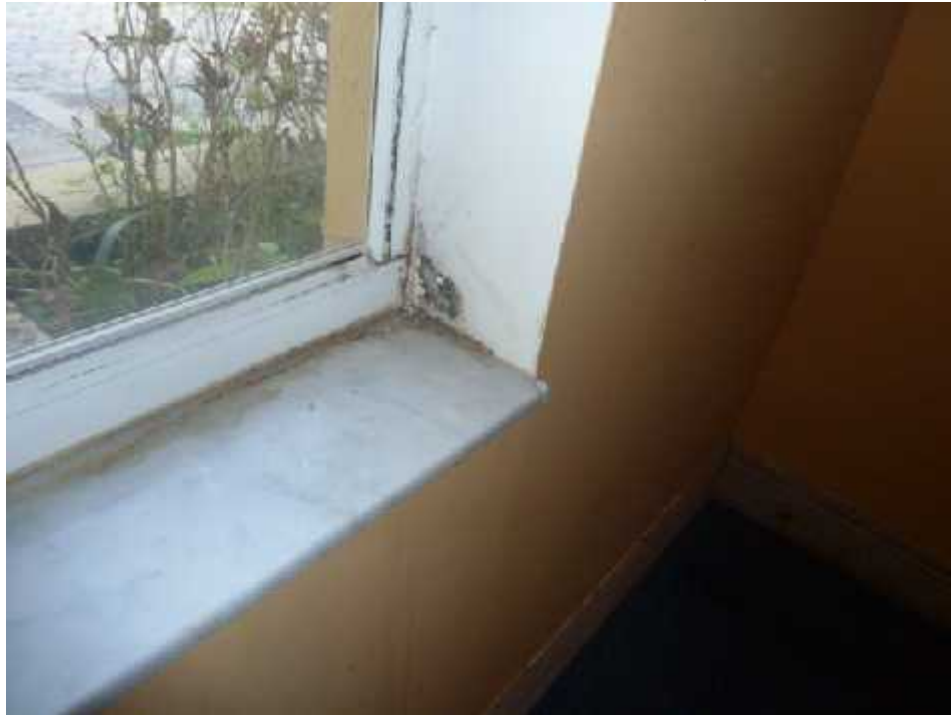
Water Damage at window in Left Front Bedroom.
