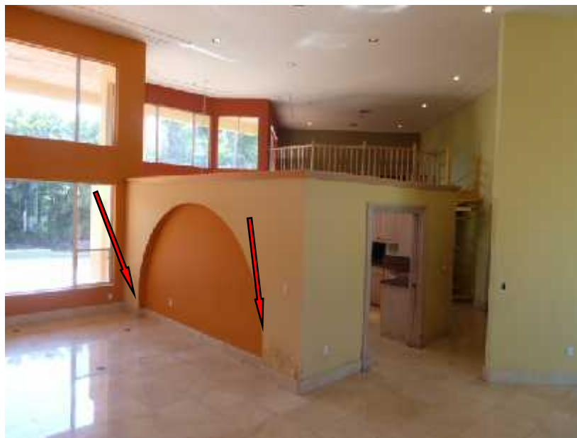
Water Damage in the Living Room
