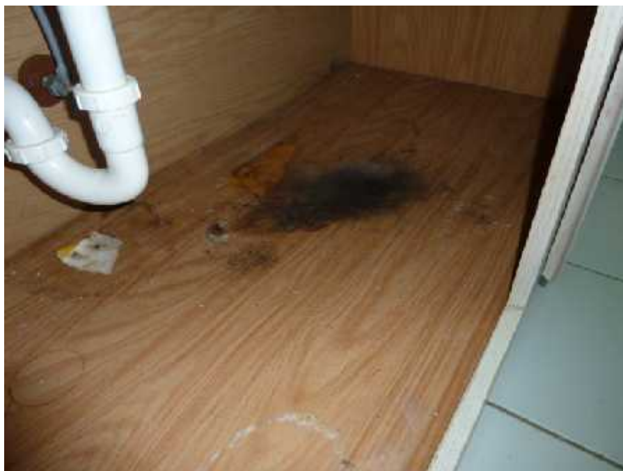
Damaged Cabinet in Utility Room
