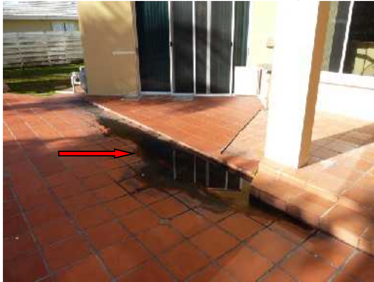
Photo: View of the Rear patio. There is a need for a drain to divert water away from the foundation. Note: Multiple layers of tiles have been installed.
