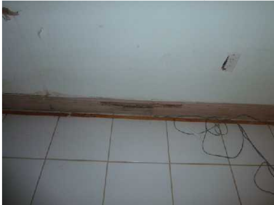
Water intrusion at Floors in Right Rear room.
