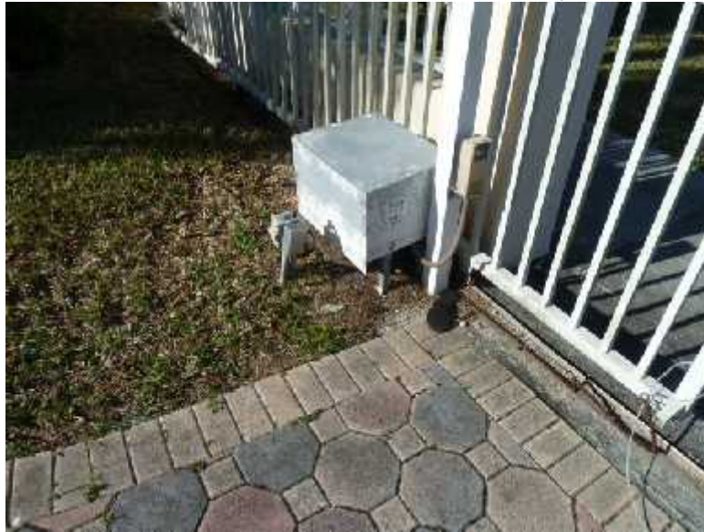
Photo: View of one of two gate openers on the property. Both openers were inoperable.
