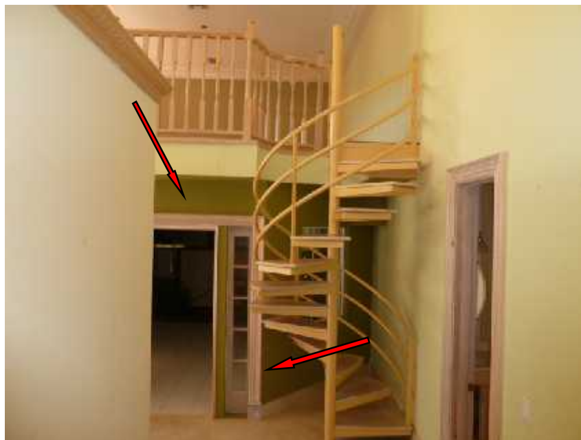
Photo: View of the loft that we believe was constructed without the approval of local municipality.
