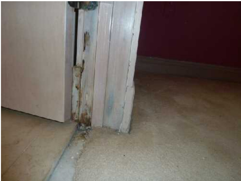
Water Damaged door and wall in Left/Center Bedroom.
