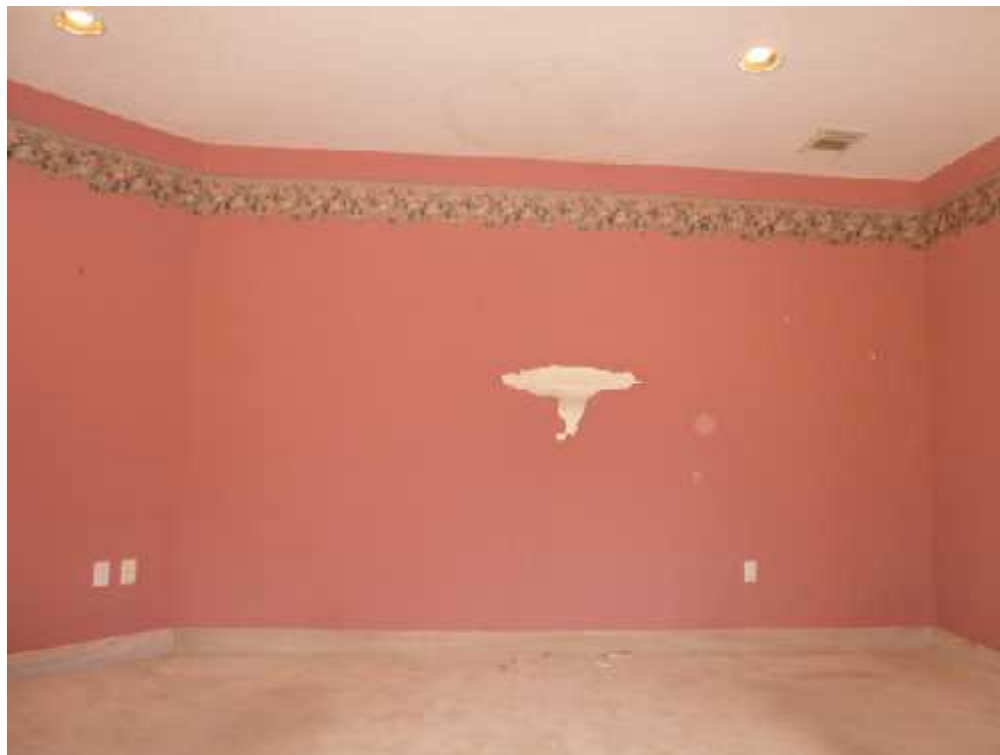
Water Damaged Ceiling and Walls in Master Bedroom
