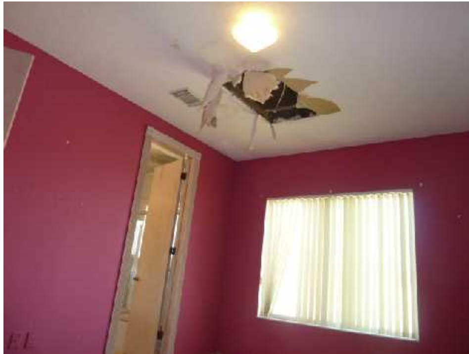
Ceiling Damage in Left/Center Bedroom
