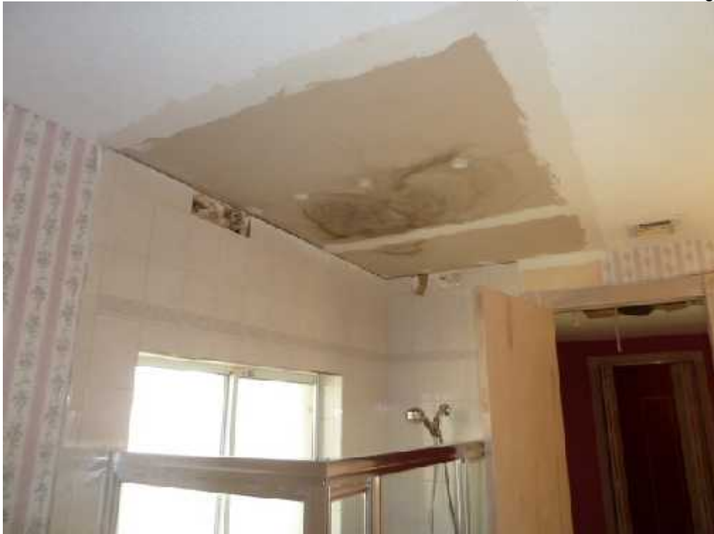
Water Damage in Hall Bathroom
