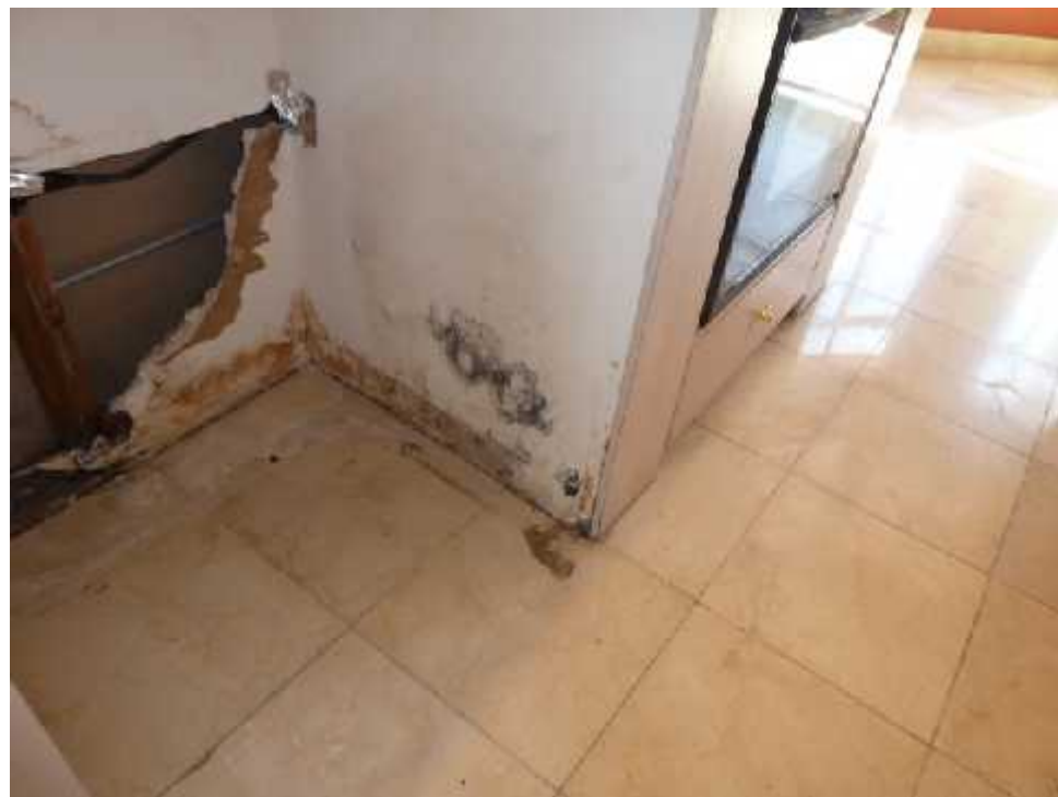
Damaged Kitchen Walls and Floor
