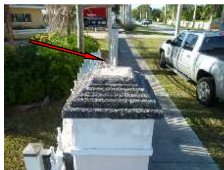
Missing Coach Lamp
