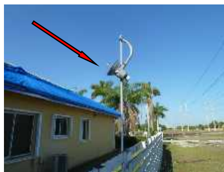
Damaged Flood Light
