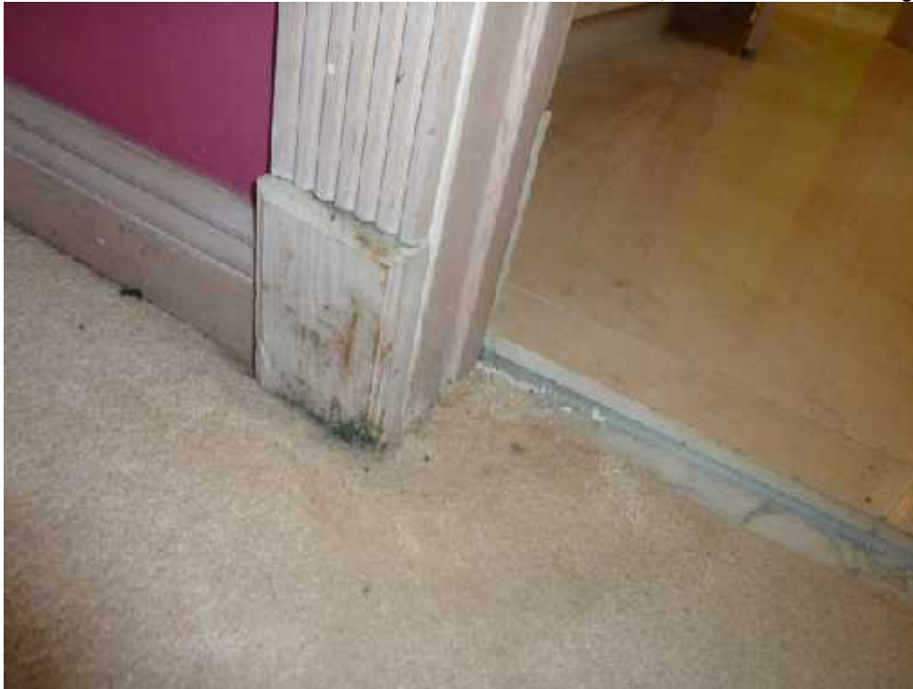
Water Damage to floor in Left/ Center Bedroom.
